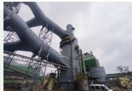
Efficient Wet Desulphurization System of Huangshi Company
