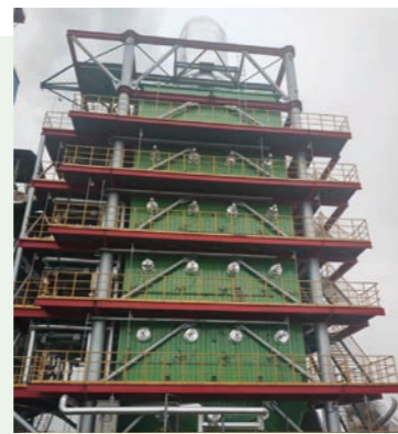
Efficient SCR Denitrification System of Daye Company
